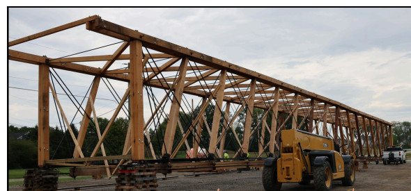
The bridge is scheduled to move less than a quarter mile away, on Sept. 5 and 6.
